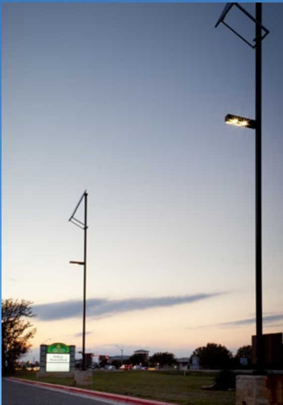
Solar Assist Streetlights - Hwy 1431
